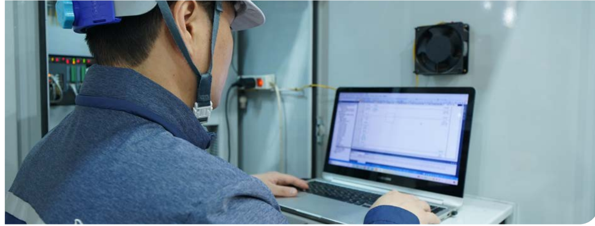
Step 1 PLC equipment control
